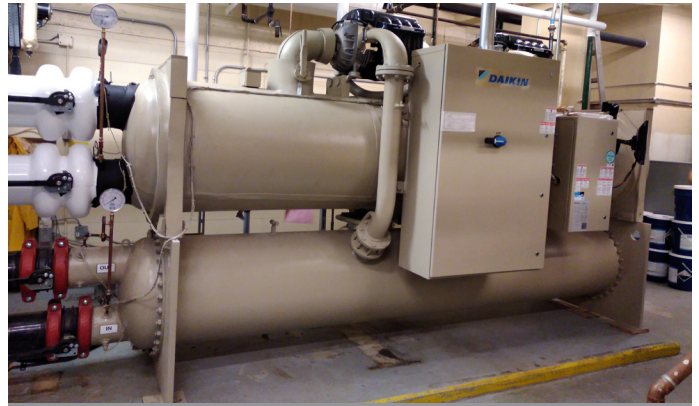
A single Daikin Magnitude WME chiller can save building owners up to $4 million over the life of the chiller.
